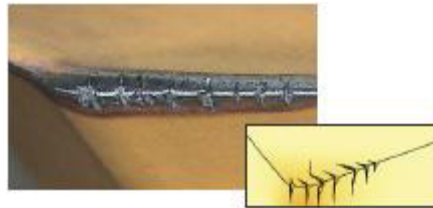
Figure 2-14: Thermal cracks – Sandvik
